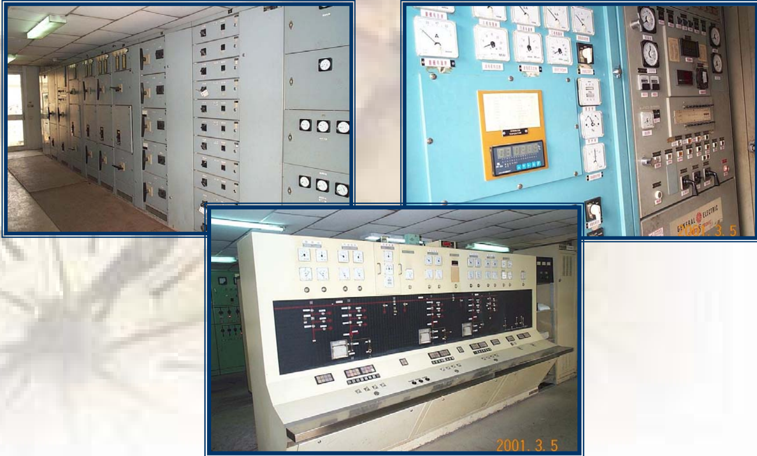
Frame 5 Complete GT Power Gen Units
